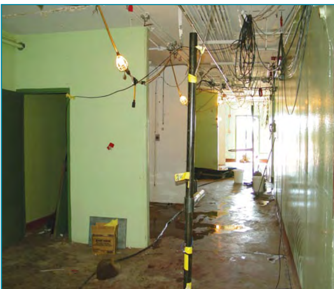
After HE pipes, fixtures, and asbestos were removed, instrumentation was attached to the exterior and interior of building 340 before a test.
