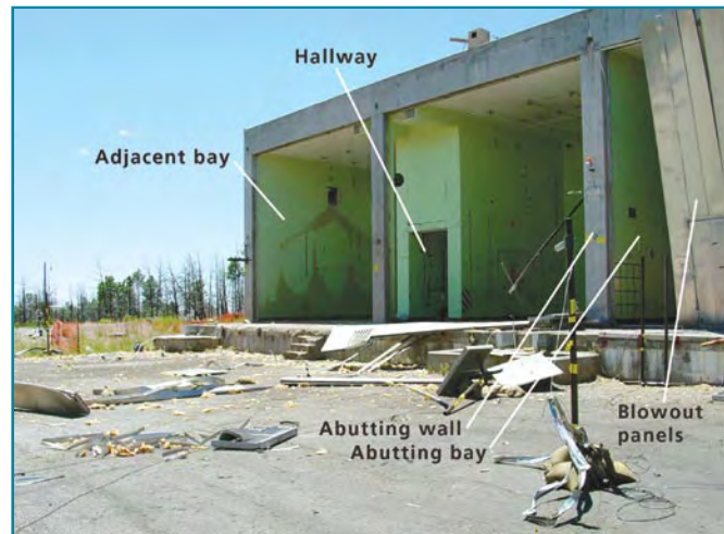
After a 25-lb test shot, blowout panels are on the ground and blowout panels in the abutting bay are damaged.
